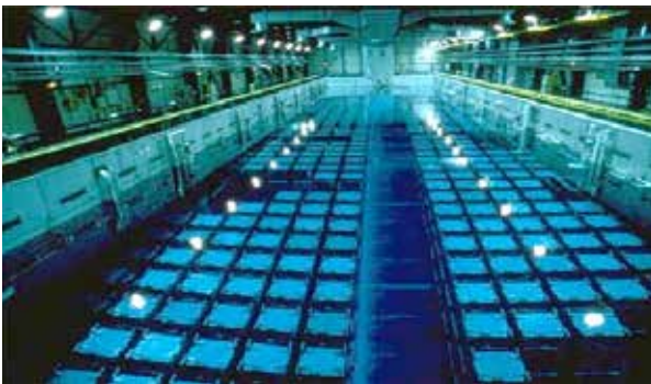
Figure 1 – Main spent fuel pool in La Hague
